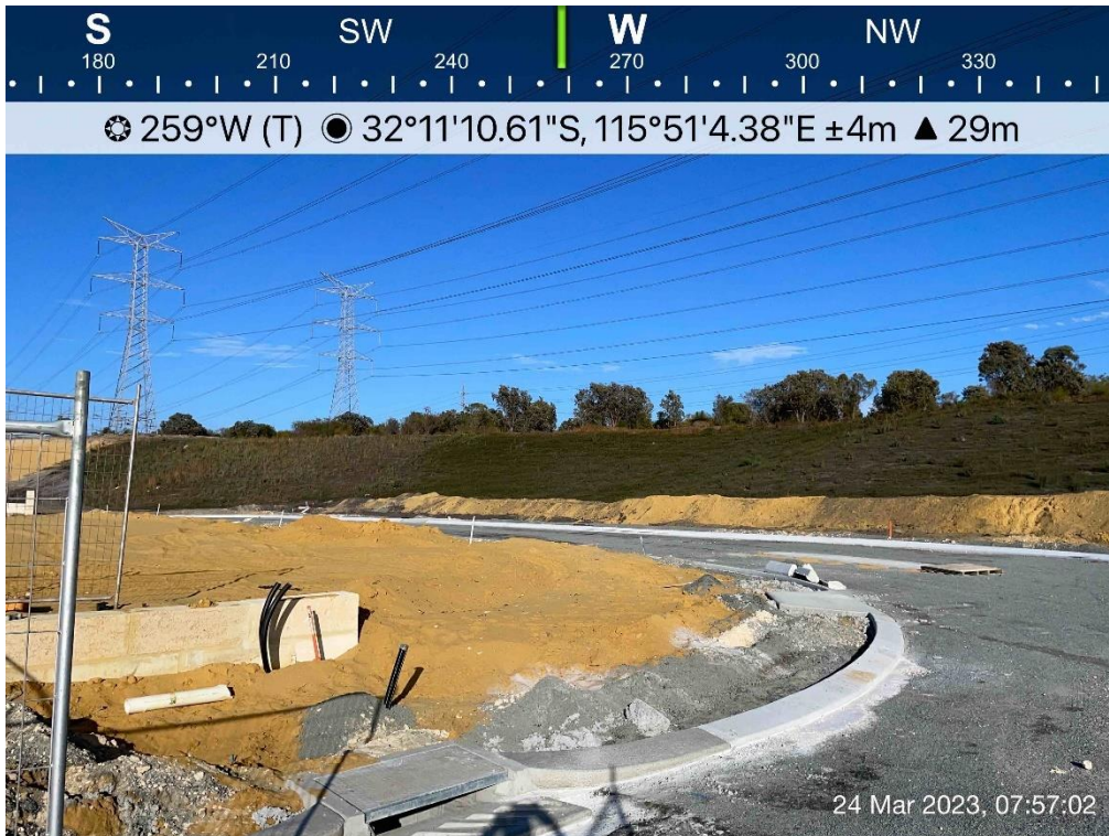
Plate 2: Residential lots within Stage 8 and APZ vegetation planting within Western Power easement.
